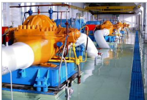
Pump station of Baltic pipeline system, Transneft
